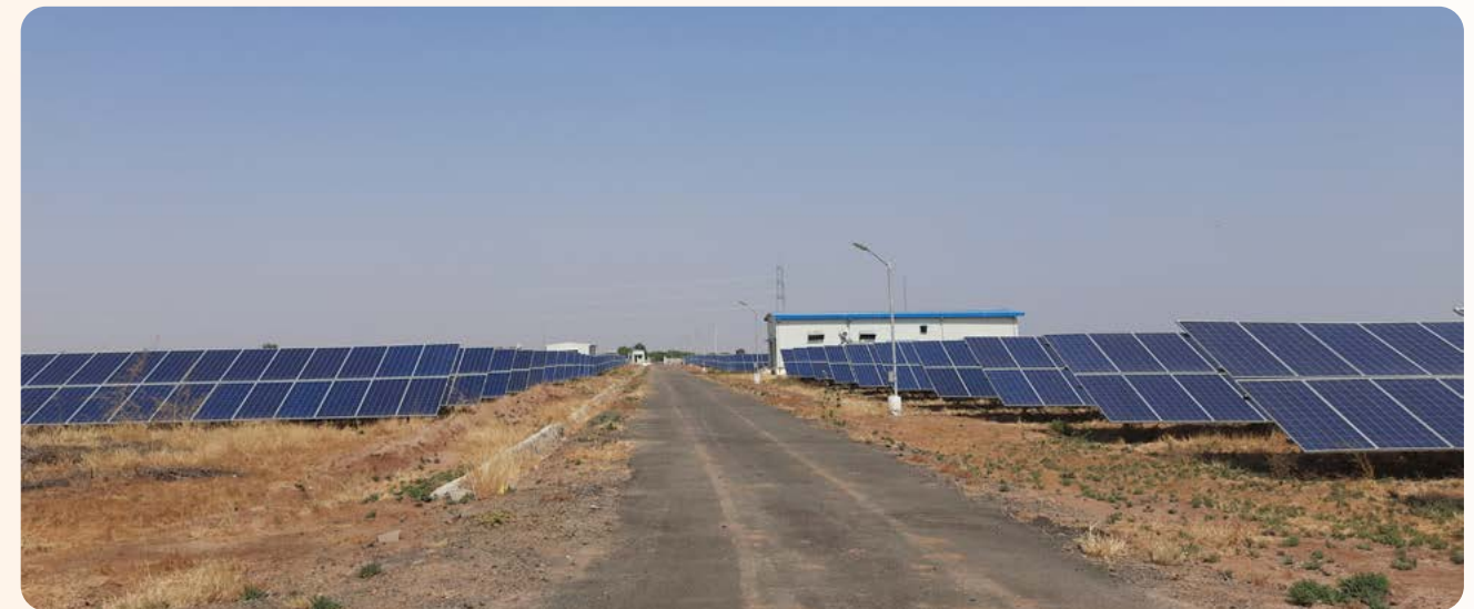
15 MW Charanka Solar Power Project
