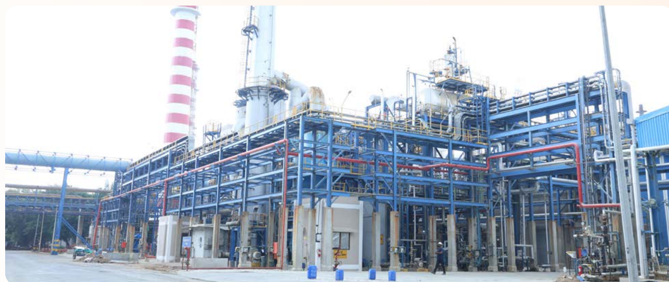
600 MTPD Sulphuric Acid-V Plant
